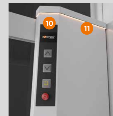
PLATFORM CONTROL PANEL
